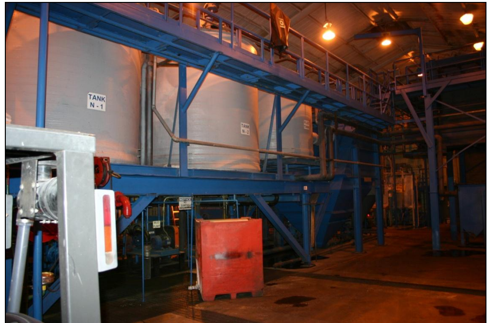
Charlotte Pipe and Foundry Water Treatment
